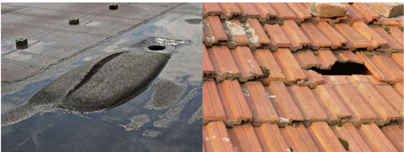
Figure 3: Typical damages on roofs ( www.bauden.at / www.hausjournal.at )
