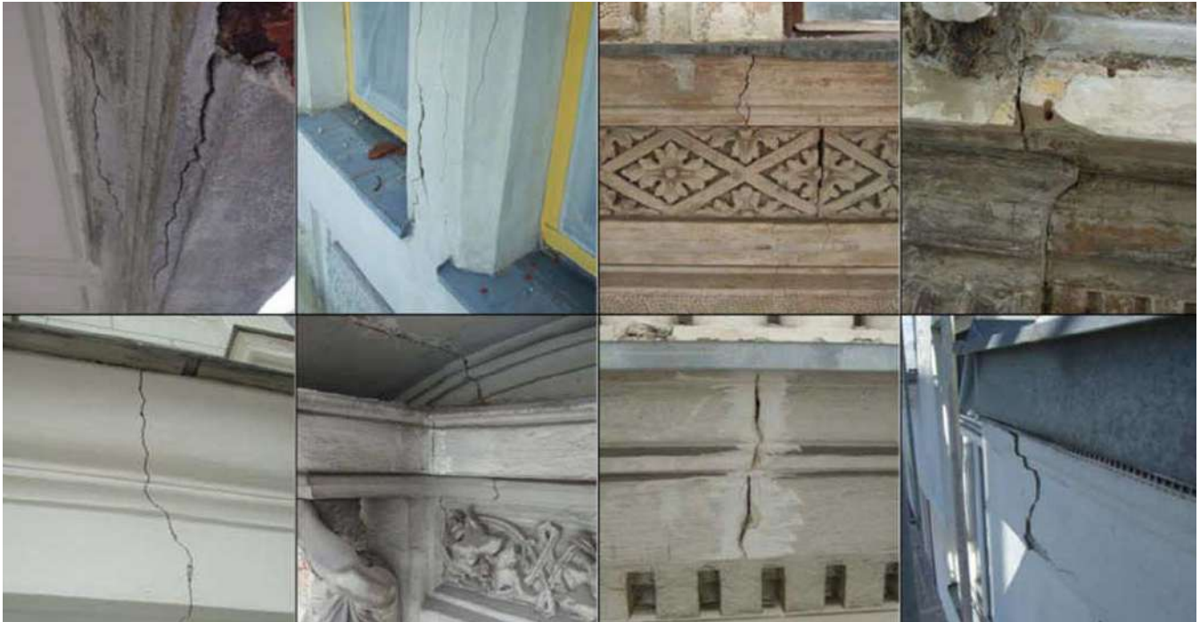
Figure 2: Typical damages on facades ( https://www.zukunft-bau.at/bauschadensberichte )
